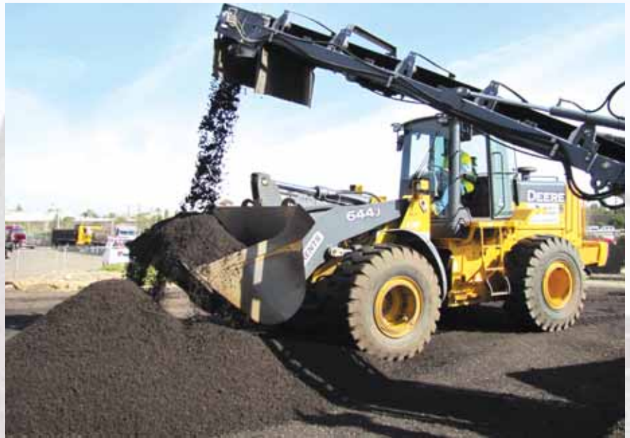
(Above) Pavement Recycling Systems takes the old road material off-site where it is crushed, screened and mixed with a recycling agent.
